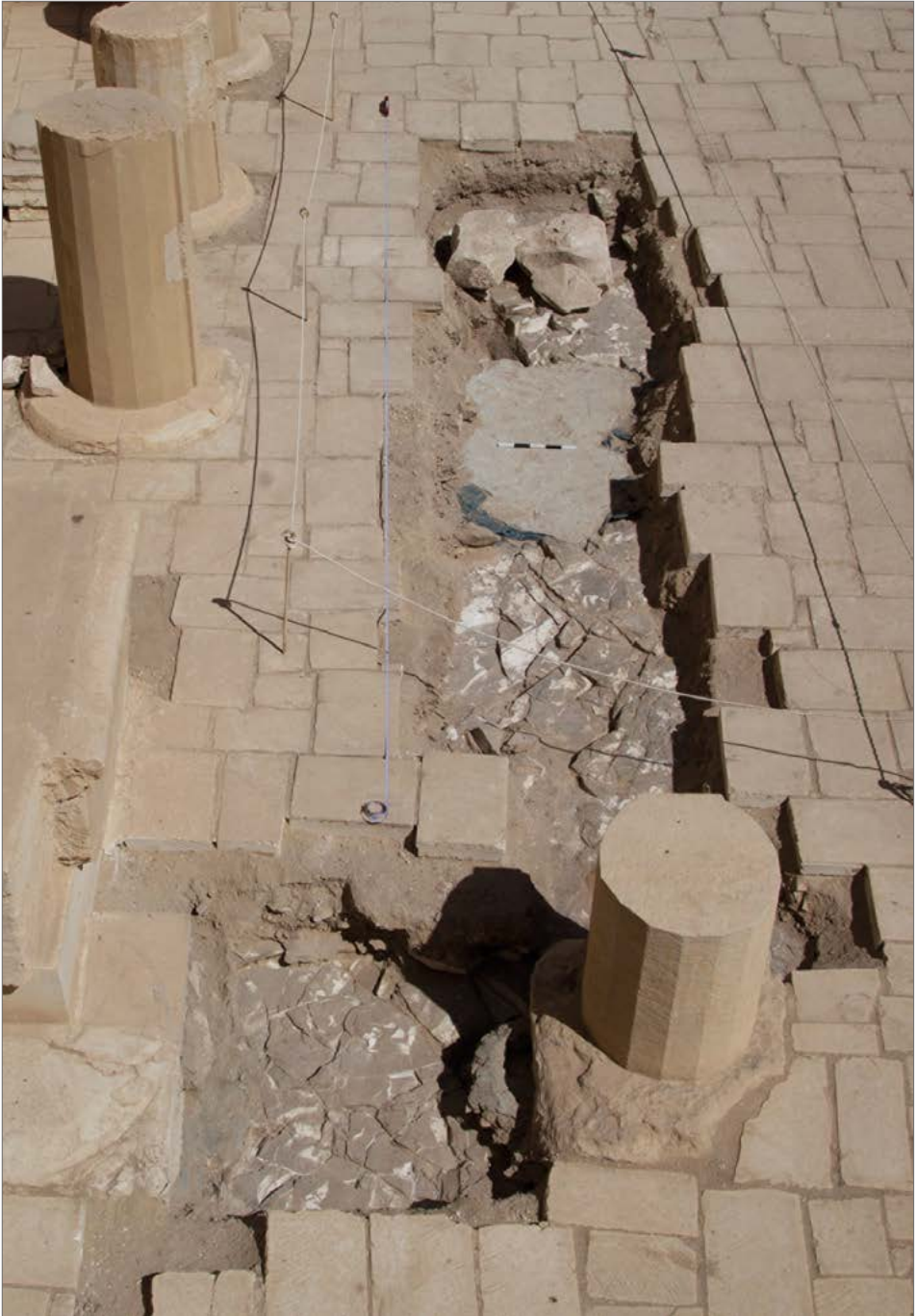
Fig. 5. General view of trench S1/15, excavated in 2015 (PCMA UW Deir el-Bahari Temple of Hatshepsut Project/photo M. Jawornicki, 2015)
